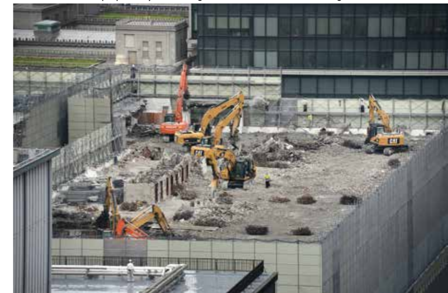
The view from the 20th On the cover of Number 1 Shimibun in 1975, and in 2015, looking from the current Club at the preparatory work being undertaken for the new building
