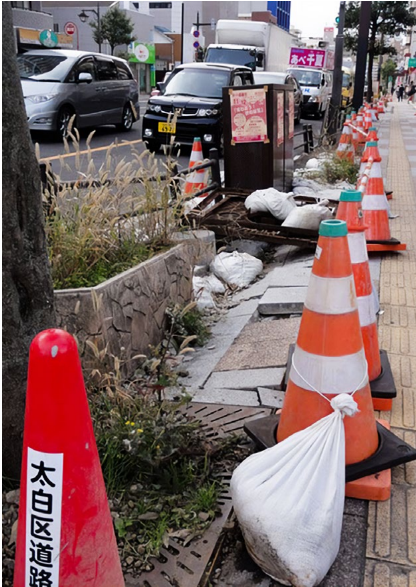
▲ Sendai city Nov. 2011: Sidewalks remain damaged and hard to navigate 8 months after the March earthquake.
