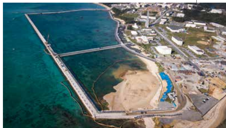
A barrier too far Landfill work off the Henoko district of Nago, Okinawa, for the relocation of the U.S. Marine Corps Futenma station. The relocation is the subject of a referendum this month. by Richard Atrero de Guzman/Nur Photo
